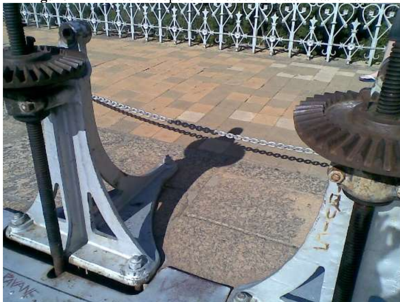
Figure 7 – Device that opens or closes the water intake valve.
