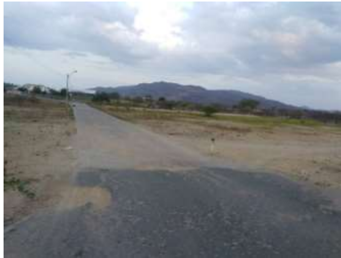
Figure 5 – Bleeding and the raceway over the bleed.
