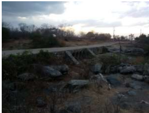
Figure 9 – Bleeding on the side of the left abutment of the dam.
